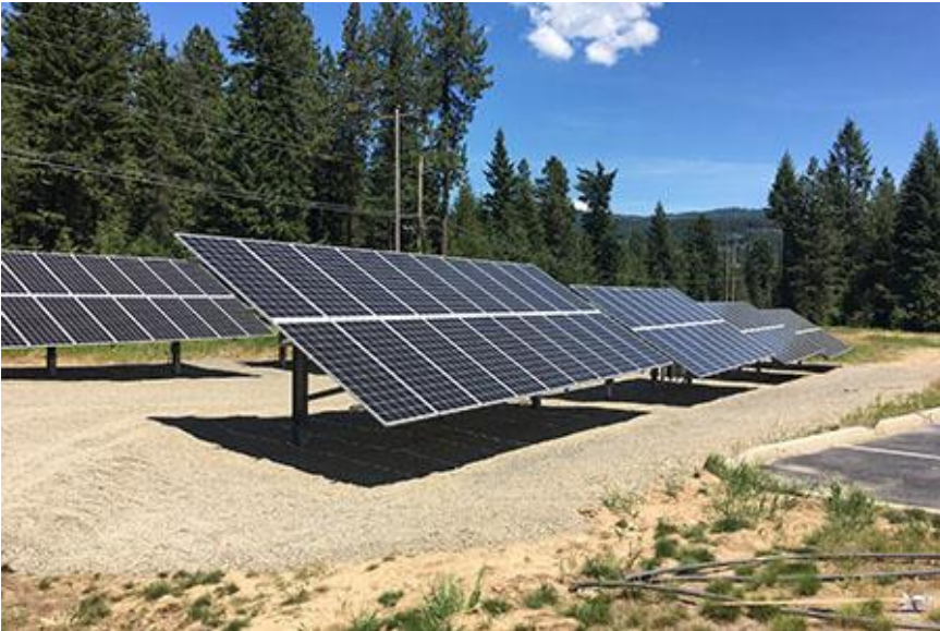
Figure 8 Ground Mounted Solar
